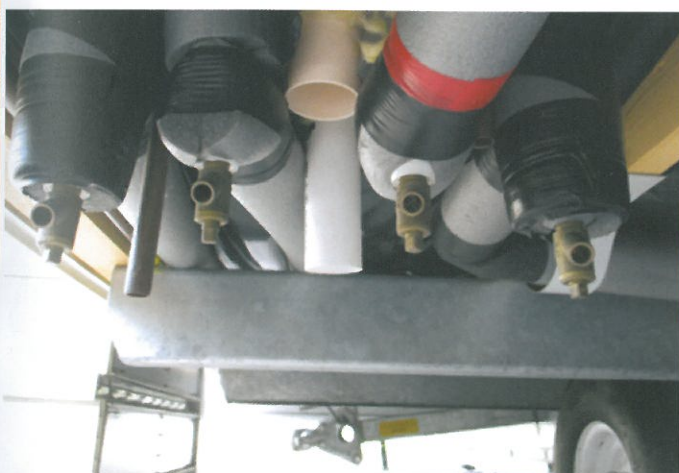
The middle two draincocks are for hot and cold water (there may be others elsewhere!). The outer two draincocks are for central heating and should not be opened.
