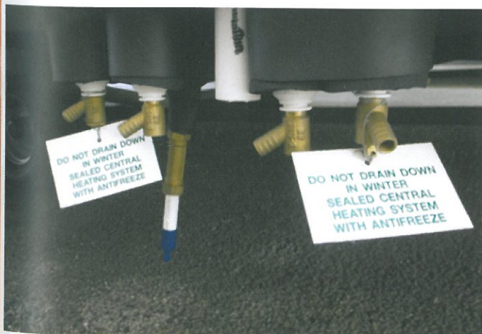
This manufacturer has helpfully labelled the central heating draincocks.
